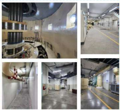
Lighting System Unit 3
